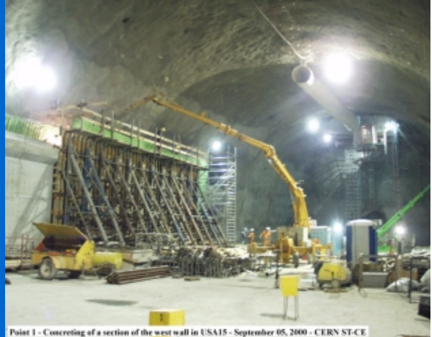
Point 1 - Concreting of a section of the west wall in USA15 - September 05, 2000 - CERN ST-CE
