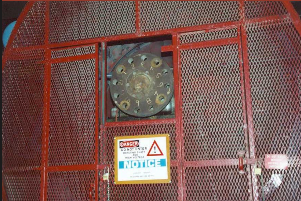
Fermilab Helium Liquifier Plant Photo by Ken Taylor
