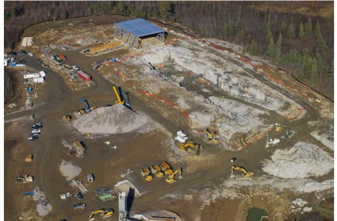
The figure shows an aerial view of the construction site in late fall 2009.
